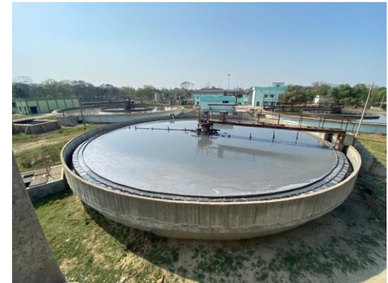
STP Jajmau process (top) and clarifier (bottom)
