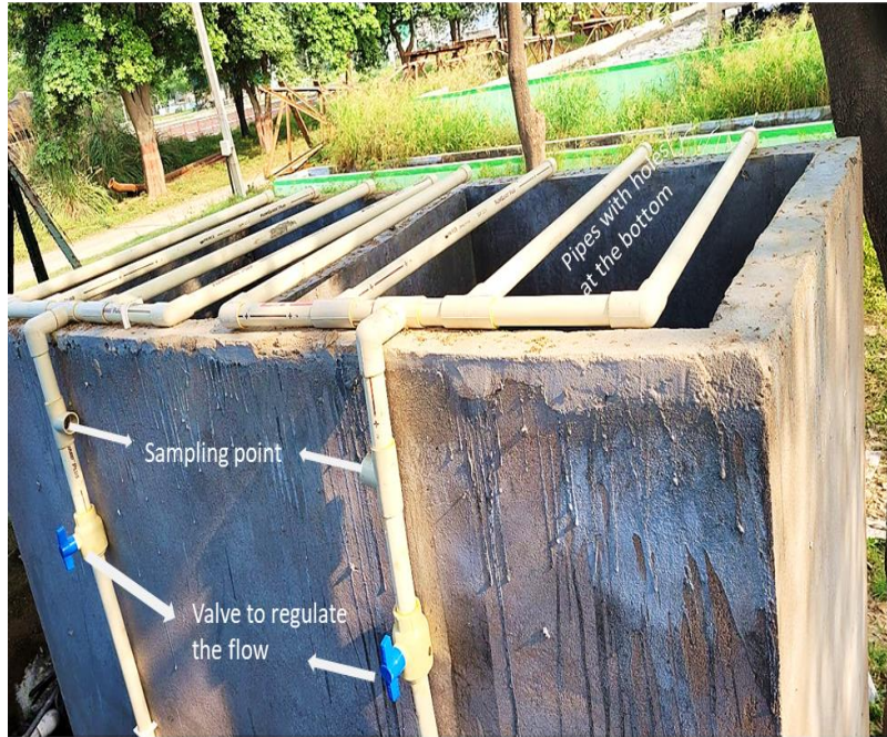
Fig. 1: Network of pipes used to distribute the influent evenly on the wetland's surface.
