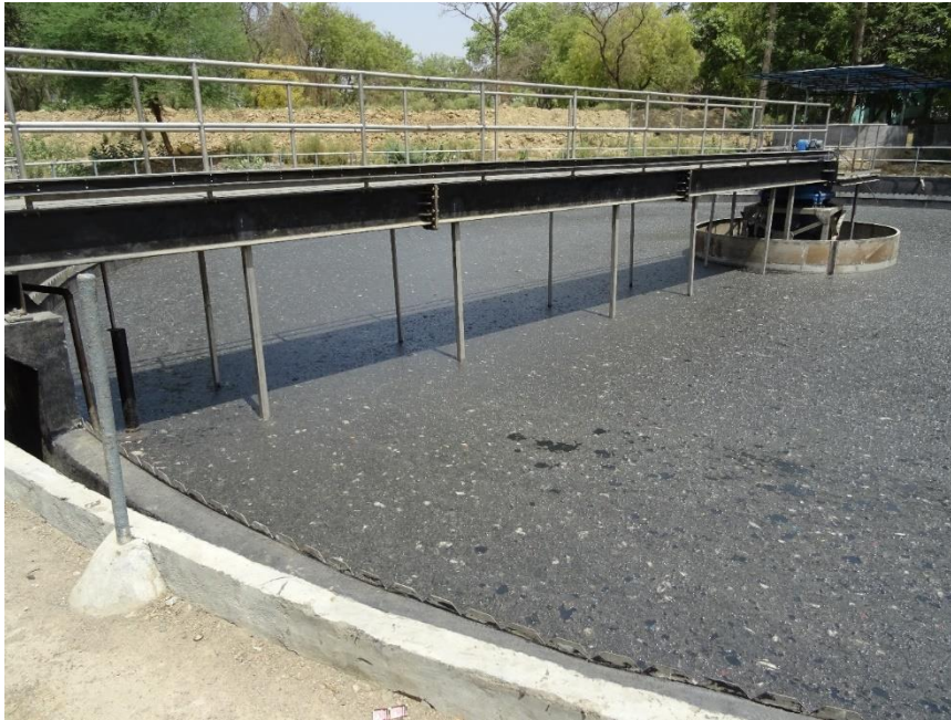
Figure 4: Sludge thickeners Line 1 Jajmau Standard Treatment Plant (STP)
