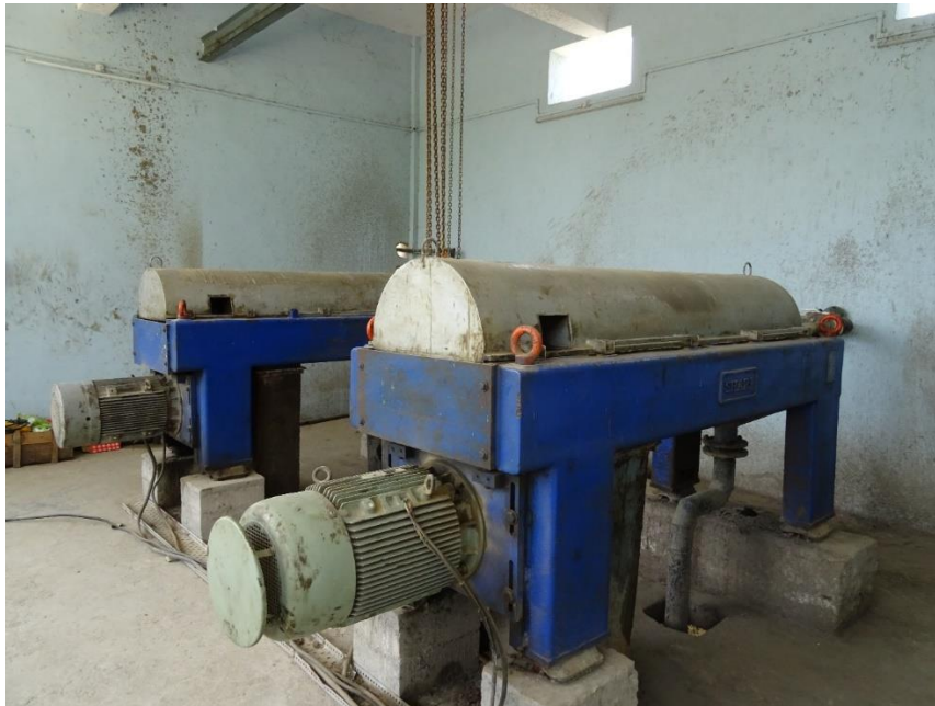
Figure 5: Sludge dewatering Line 2
